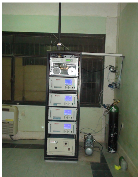
Figure 2: All instruments in the South Valley station
